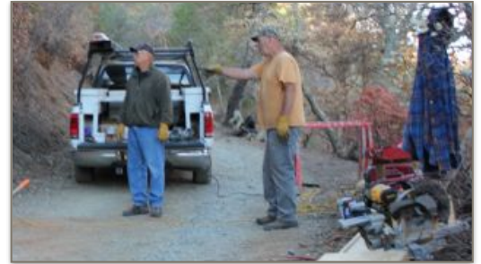
Pat and his crew building the exit stairs on the Cruse round.
